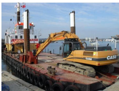
Doreen Dorward, following £80,000 refit, and state of the art Case CX350 excavator with RTK GPS dredge system.
